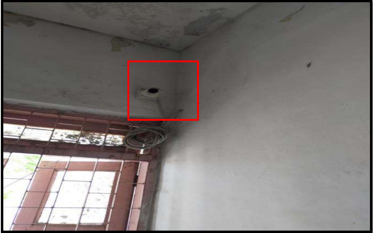
CCTV camera inside the Examination Department
