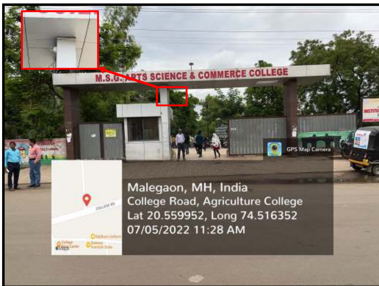
CCTV Camera at College Gate
